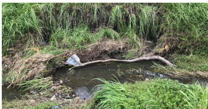
倒木と護岸の崩れ
